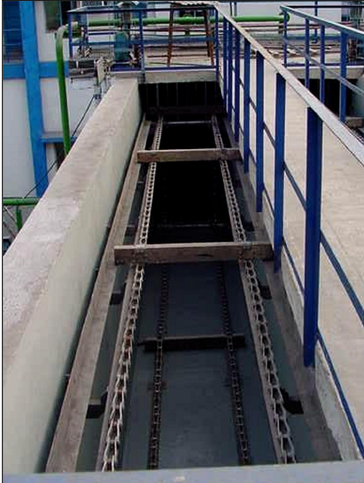
API Oil Separator
