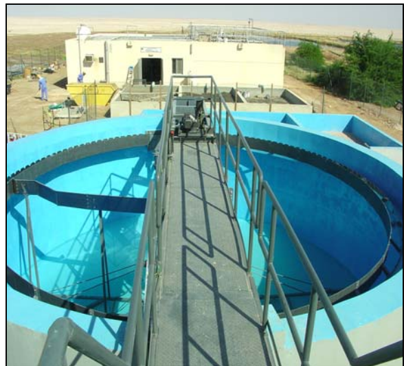
Central Driven Bridge Mounted Clarifier
