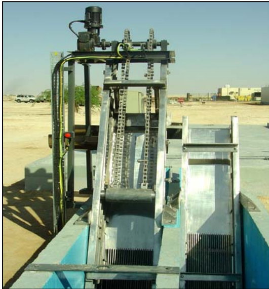
Mechanical Inclined Bar Screen
