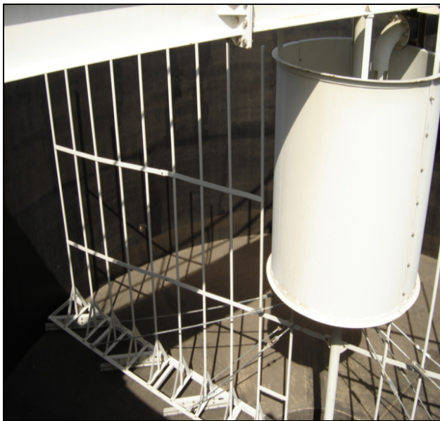
Picket Fence Arrangement in Sludge Thickener
